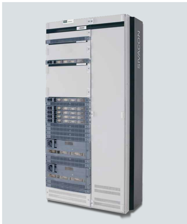
The section for switch disconnectors with 3NJ6 LV HRC fuses is suitable for up to 35 tap-off units in a fused system.
