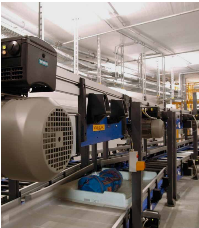
Whether for industrial applications or infrastructure, energy costs can be lowered thanks to the reactive power compensation.
